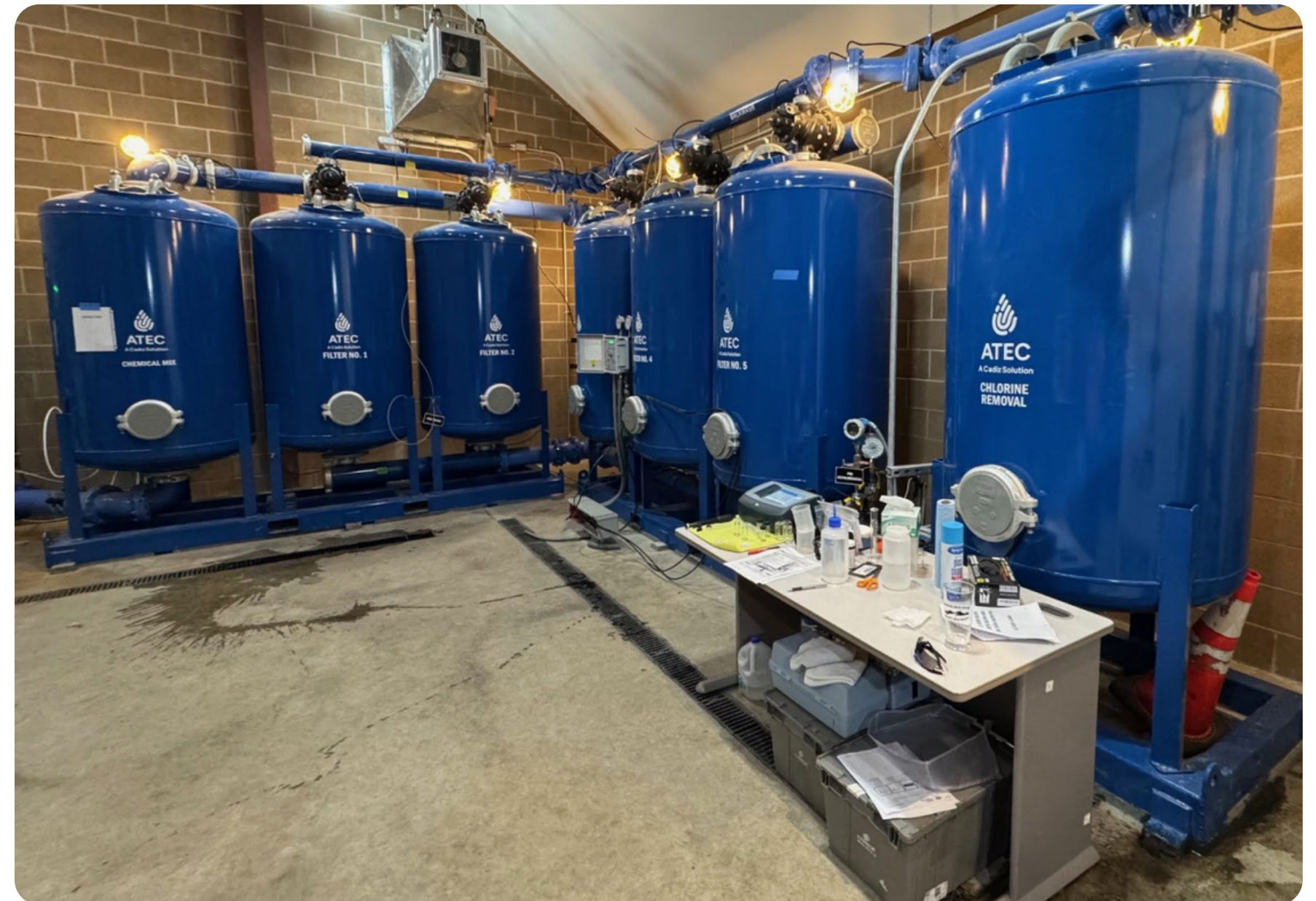
Snoqualmie Pass Utility District treatment system for arsenic removal
