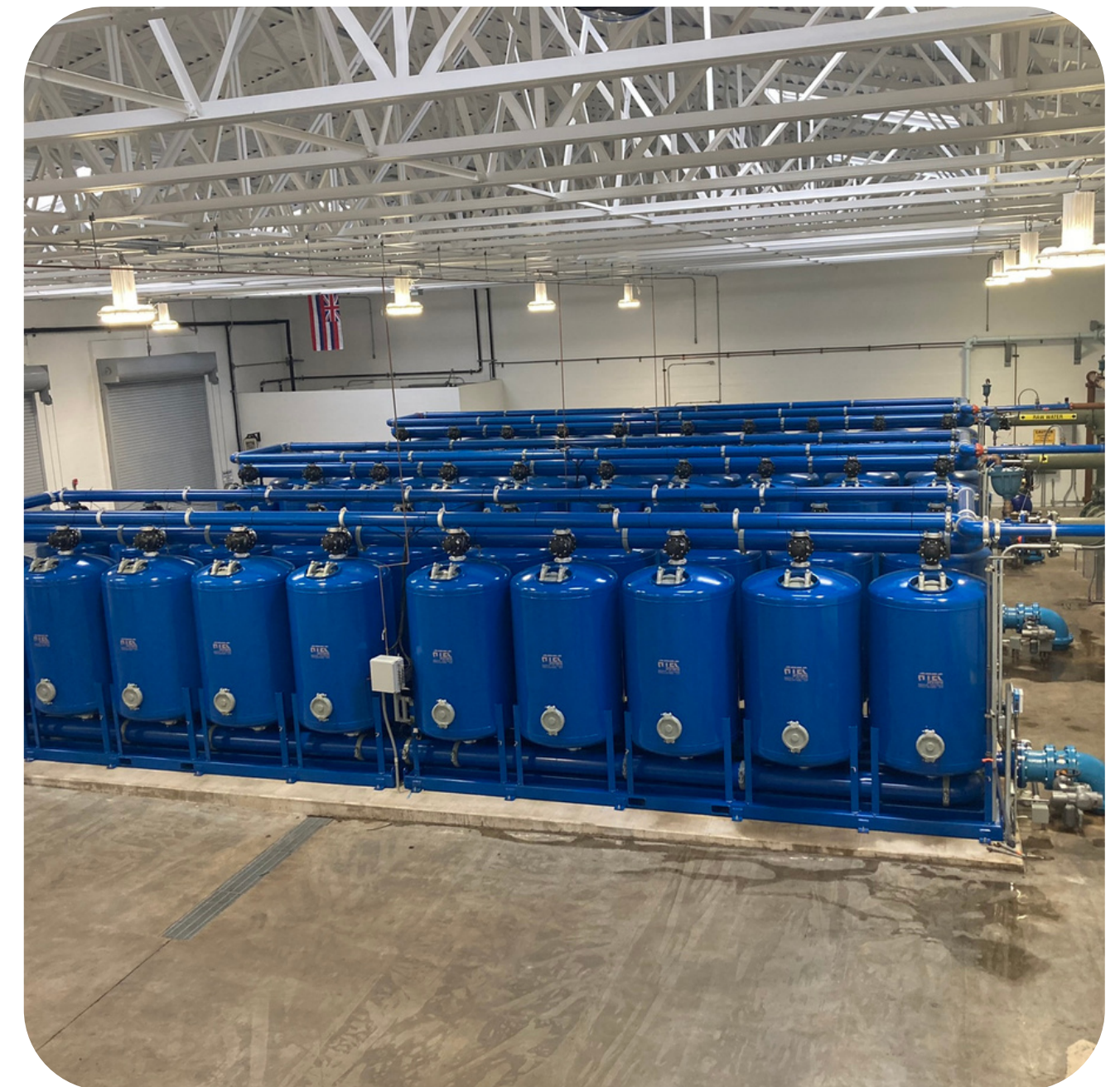
This 15 mgd (60 MLD) water treatment plant in Ridgefield WA has been in operation since 2019.
