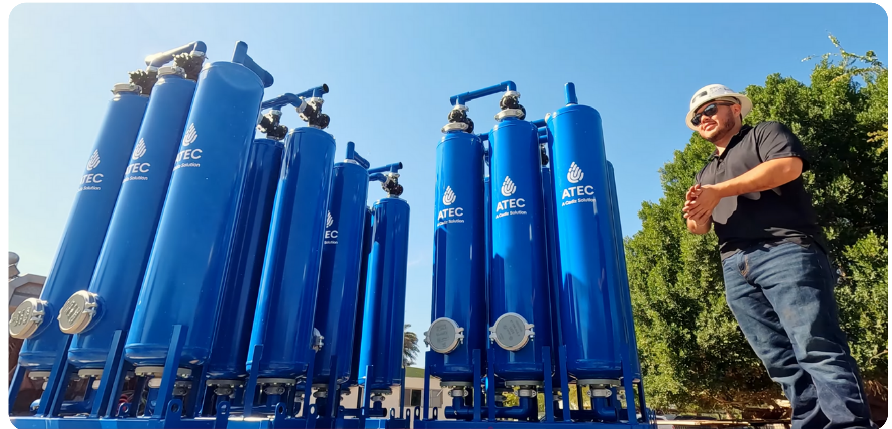
ATEC's OCF arsenic treatment system delivering reliable compliance for the Torres Martinez community in the Eastern Coachella Valley.
